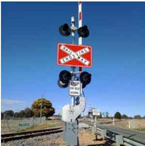
4SITE Infrastructure Monitoring System, monitors status of remote equipment and alert staff to servicing
